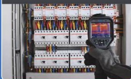
ELECTRIC PANEL INSPECTION
