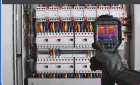
ELECTRIC PANEL INSPECTION
