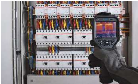
Electric Panel Inspection
