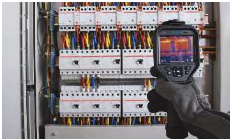
Electric Panel Inspection
